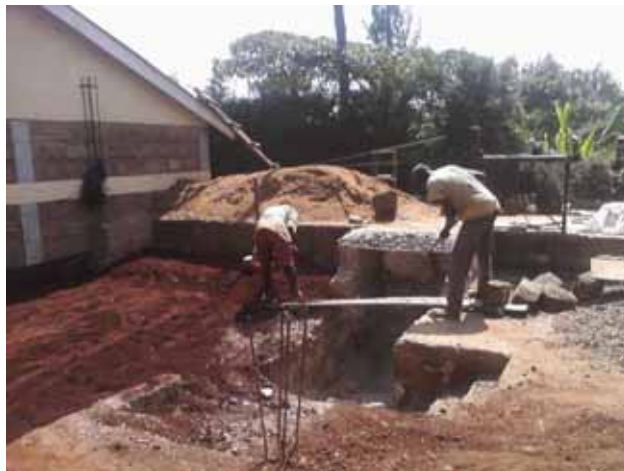
Workers digging foundations and sewers for new bathrooms at the Kihumo Head Start school
